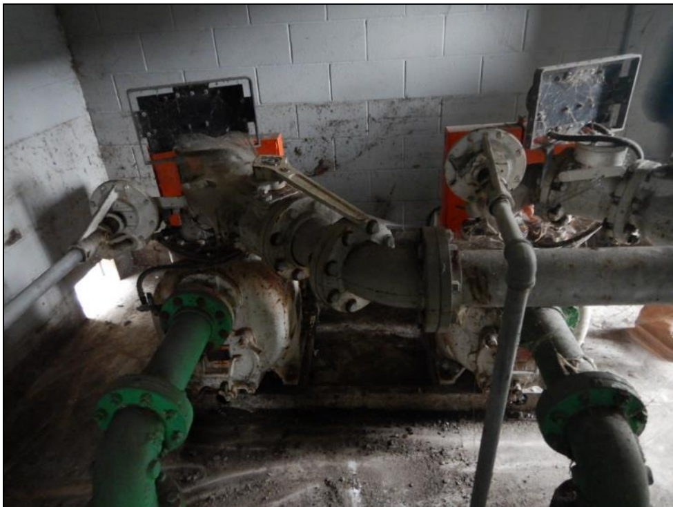
Photograph 2. Influent pump station (lower capacity pumps).
