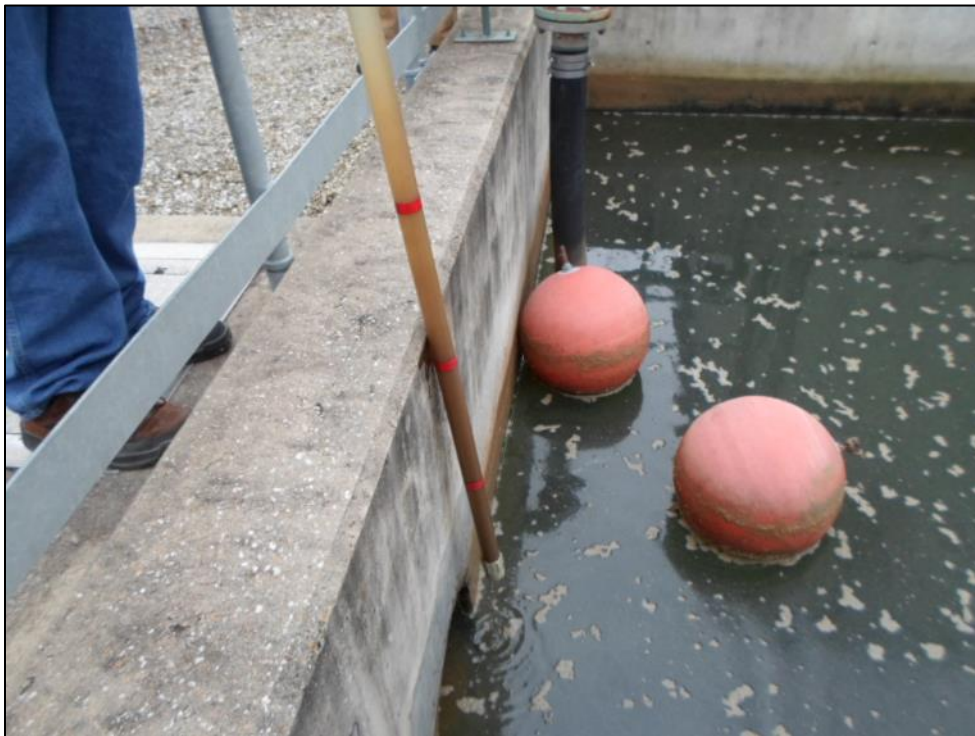
Photograph 10. Sludge judge measurement taken from the post-aeration basin.
