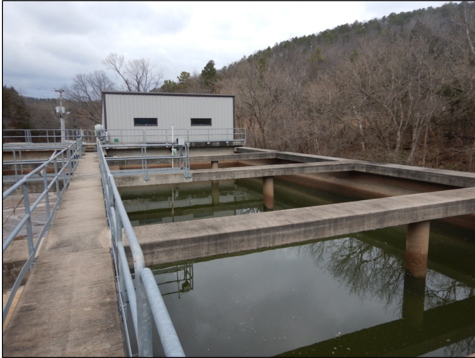
Photograph 7. The eastern SBR basin during the settle mode.
