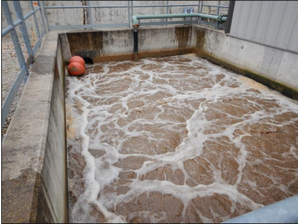
Photograph 9. Post-aeration basin while aerators are on.
