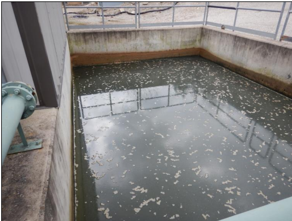
Photograph 8. Post-aeration basin while aerators are off.
