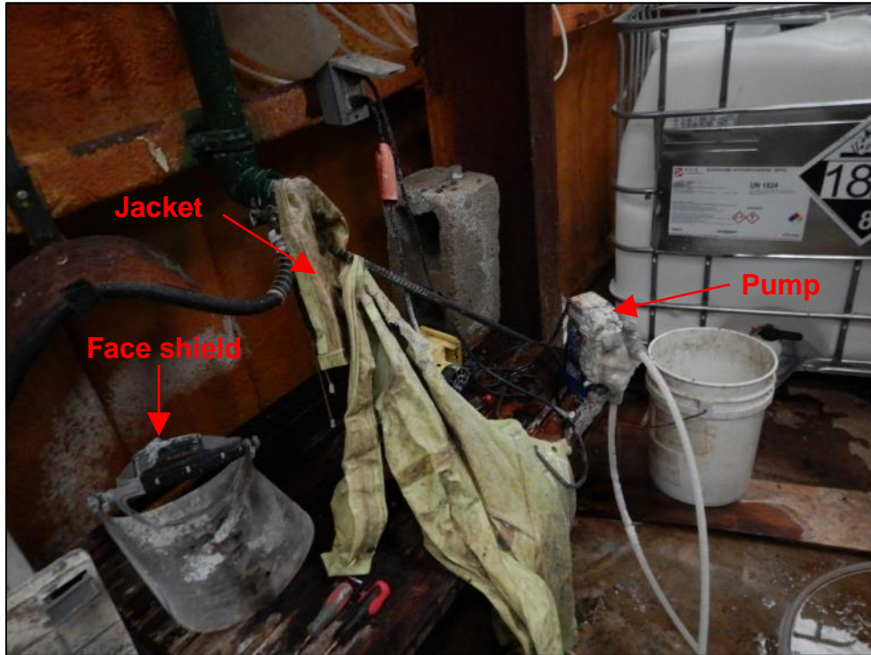
Photograph 11. The sodium hydroxide chemical feed pump was spraying 50% sodium hydroxide solution to the surrounding area, including the jacket and face shield used to handling the sodium hydroxide.
