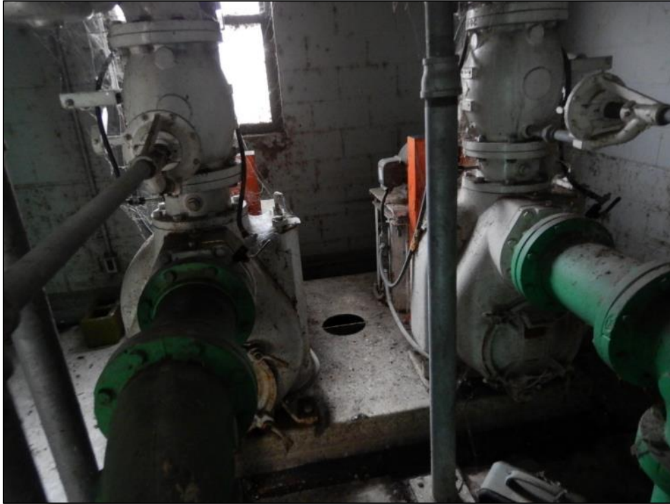
Photograph 3. Influent pump station (higher capacity pumps).
