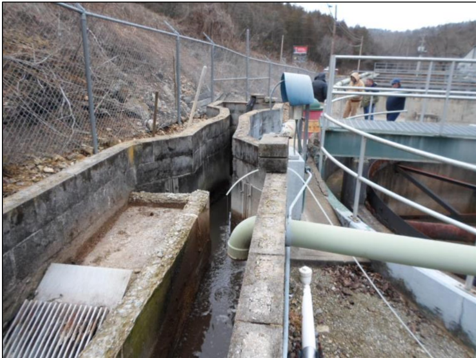
Photograph 4. Influent channel prior to SBRs. The decommissioned clarifier is to the right-hand side.
